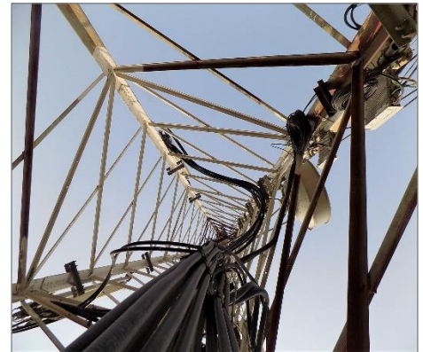
(c) Optic Cables
