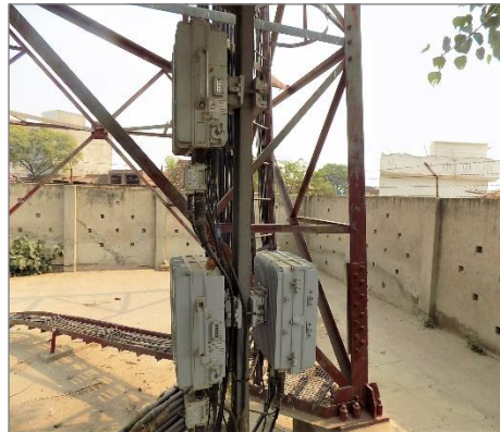
(b) RRU's attached to Shelter
