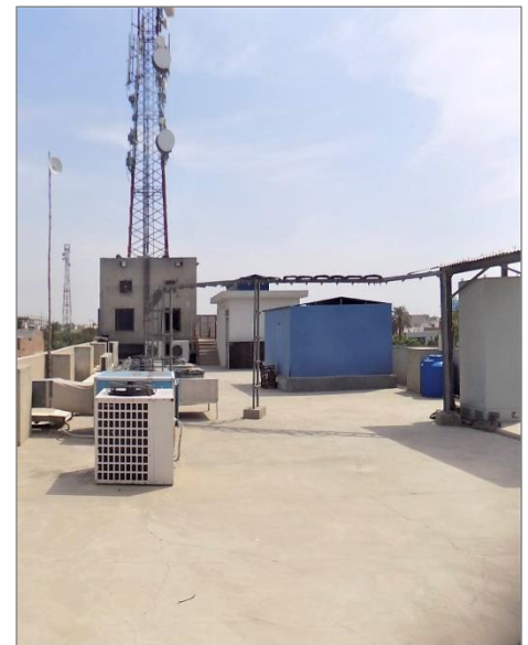
(c) Rooftop Telecom Site
